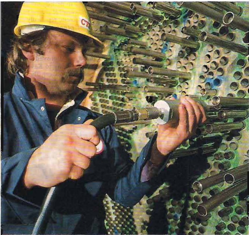
4. Tube relining may help older powerplants stay competitive by maintaining heat-transfer efficiencies and avoiding costly component replacement
