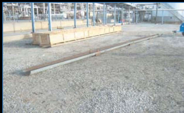
Figure 1. A 1 ft diameter pipe was cut in half. Two boxes of Hastelloy C-276 liners (in background) were loaded into the pipe and lifted by crane to 40 ft elevation for installation by CTI crew.
